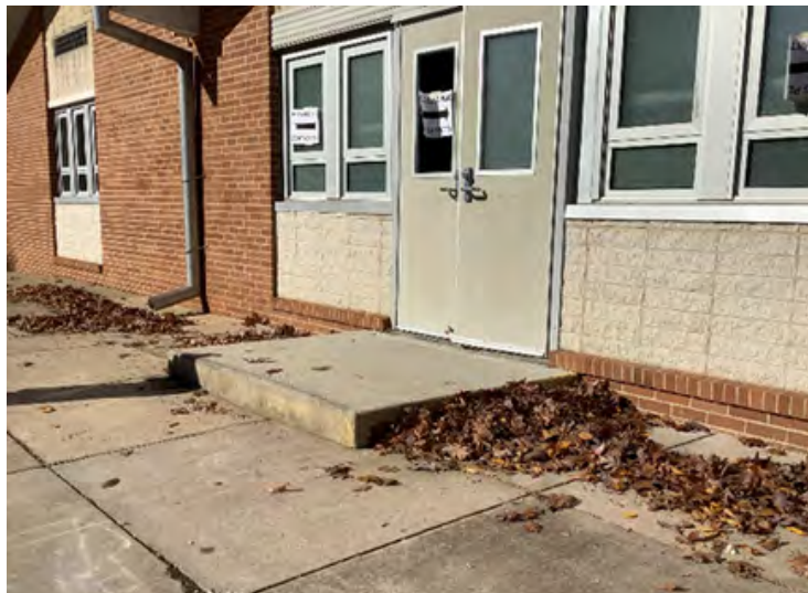
Entrance with 7" step, no ramp, cracked surface. (Polling Place: Maclary Elementary School)
