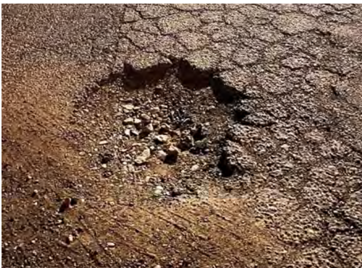
Cracks and holes in pavement. (Polling Place: Eden Support Services)
