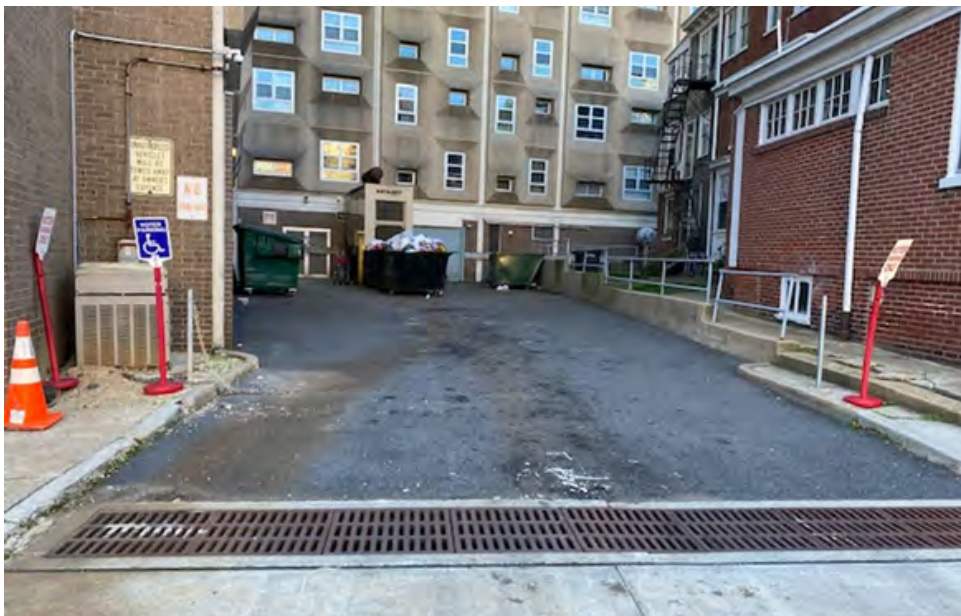
The single parking spot marked as accessible is located in the service alley near the dumpsters; there are no surface markings, and there was debris and a drainage grate between the spot and a crumbling, high curb. The entrance door was less than 32” wide and was propped open with a chair, further blocking the entrance. (Polling Place: Luther Towers)
