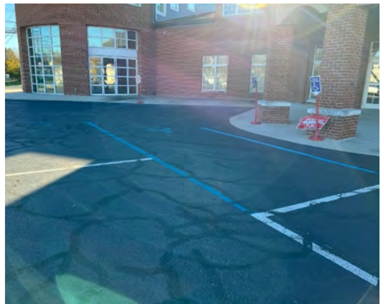
No access aisle. (Polling Place: Townsend Fire Hall)
