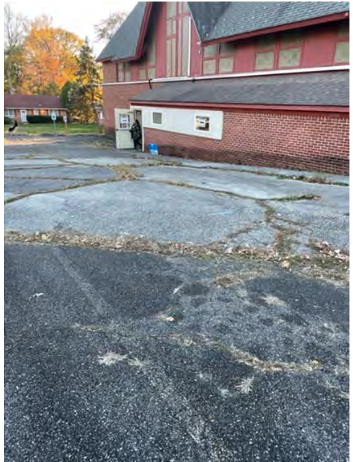
Steep slope, uneven surface. (Polling Place: Hillcrest Bellefonte Methodist Church)
