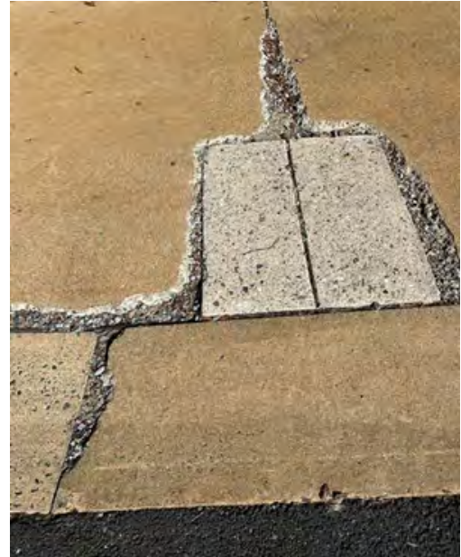
Cracked, crumbling pavement. (Polling Place: Activity Center at Hockessin PAL)
