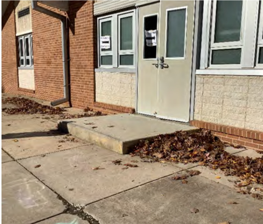
7" step, no ramp, cracked surface. (Polling Place: Maclary Elementary School)
