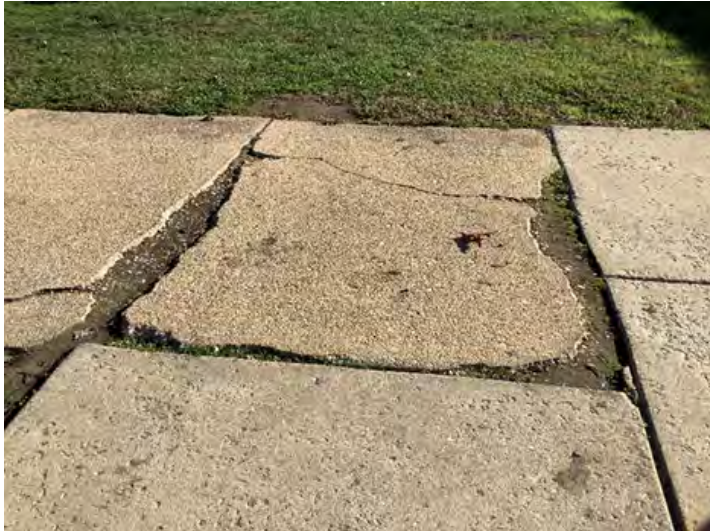
Cracked, crumbling pavement. (Polling Place: Newark High School)
