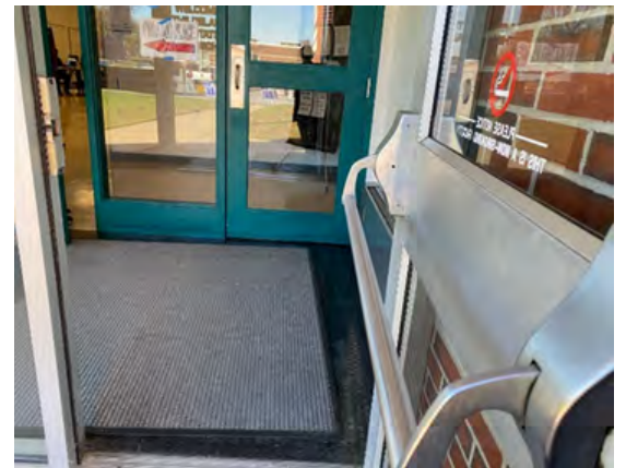
Door width narrows to 27 inches when open because of door handle. (Polling Place: State Fire School)
