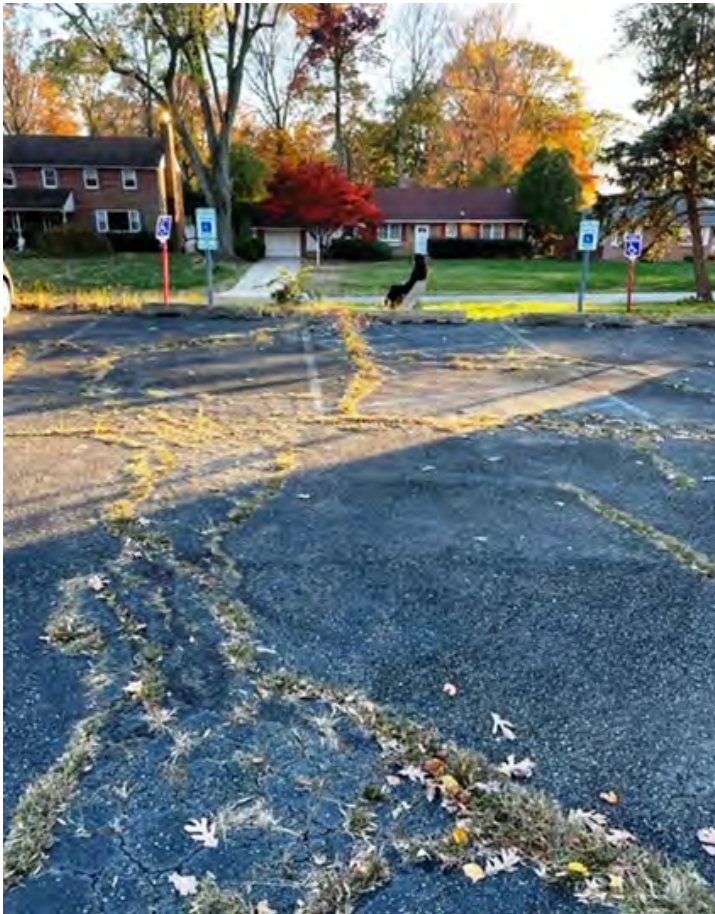
Cracked surface with debris. (Polling Place: Hillcrest Bellefonte Methodist Church)
