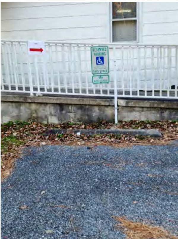
Loose gravel, no access aisle, sign too low. (Polling Place: Redden Community Center)
