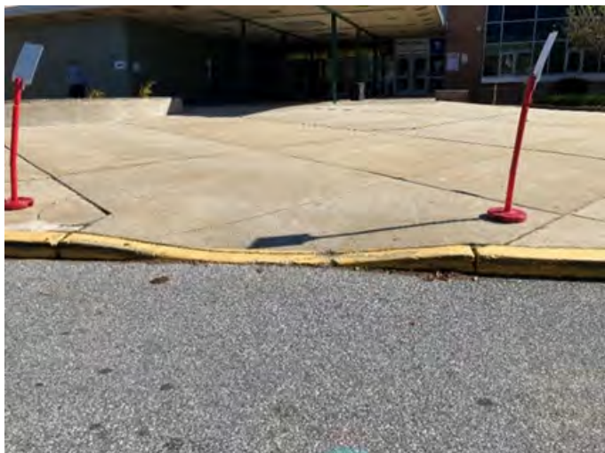
Crumbling curb cut, less than 36" wide. (Polling Place: Cab Calloway School for the Arts)
