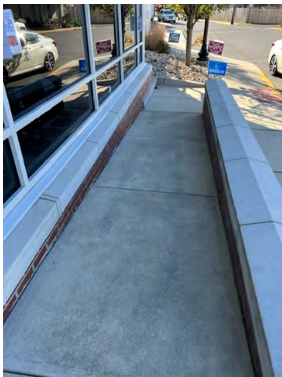
Ramp without any rail. (Polling Place: Clayton Fire Hall)
