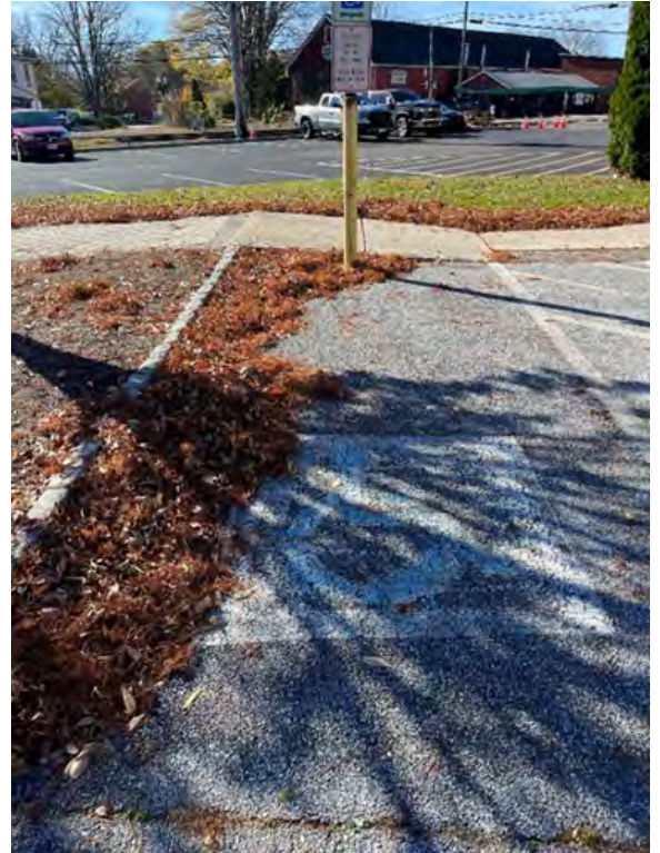
Space and access aisle too narrow. (Polling Place: Hockessin Fire Co.)
