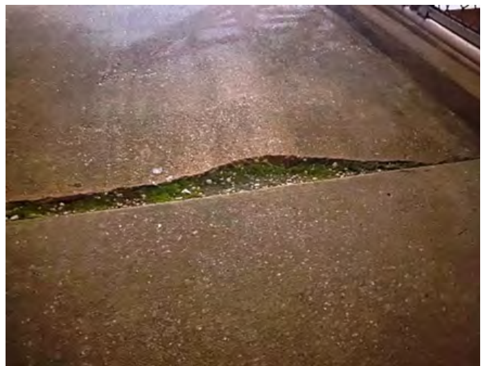
Cracked, crumbling sidewalk. (Polling Place: Eden Support Services)
